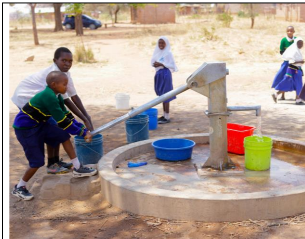
Dip well-constructed by HAPA in Kipunda Primary school in Ikungi DC, under Wibia e.V support in 2022
